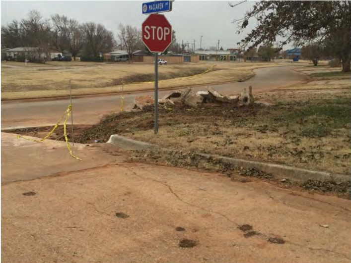
Photo 10: View of infrastructure construction on south side of intersection of S Janeway Avenue and McClaren Street.
