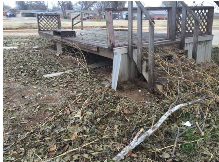
Photo 32: View of remaining residential infrastructure near intersection of S Janeway Avenue and SW 13th Street.
