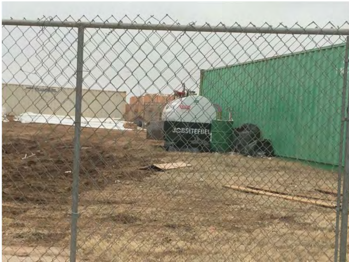
Photo 27: View of construction staging area and AST located near intersection of SW 14th Street and Yule Drive.
