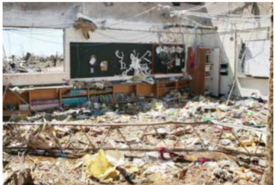
Figure 3: Damages at Plaza Tower Elementary
